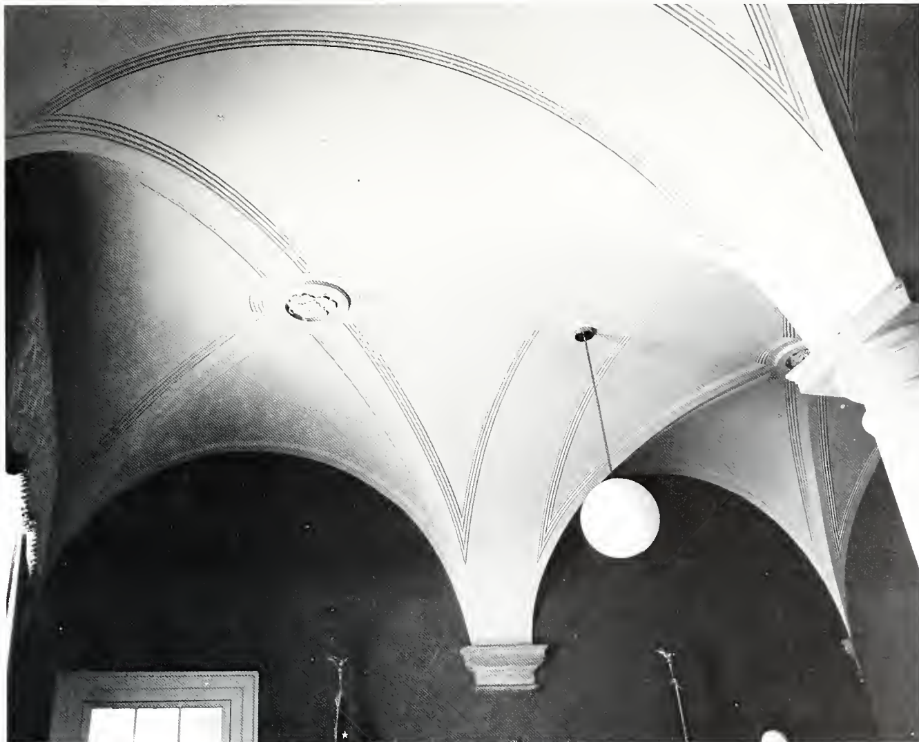
4. Groin vaulted ceiling of Governor's Office. The central stone column supports the masonry vaults, which were used to make the first floor fireproof.
