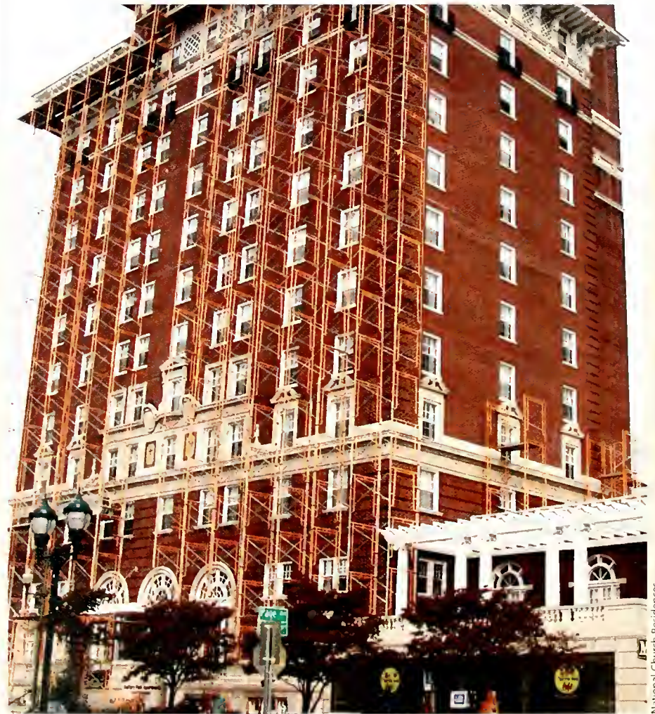
Scaffolding on Battery Park Apartments in downtown Asheville during National Church Residences' recent renovation of the 122-unit former hotel.
