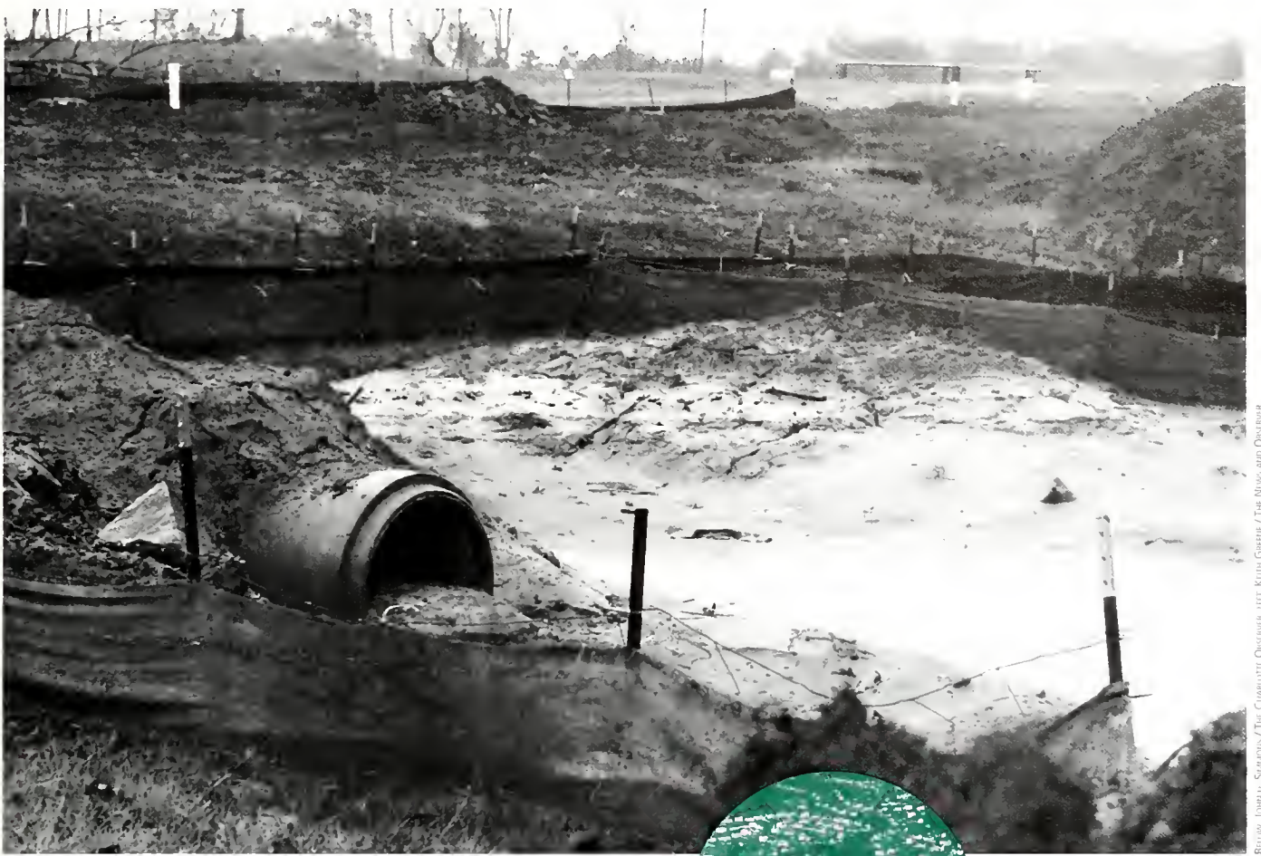
Stormwater runoff caused by the construction of a residential development.
