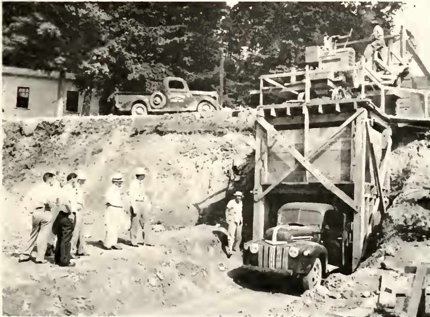
The crusher-bin-loading platform which will enable Asheboro to effect a considerable saving in providing a good stone base for its unpaved streets.
